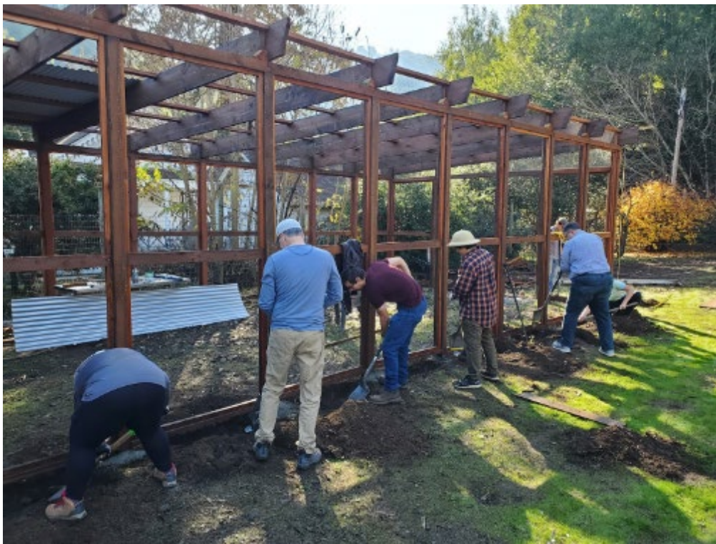
Figure 155. Digging a trench at the base of the new chicken coop just to the west of the white house during the Fall 2024 work project.
