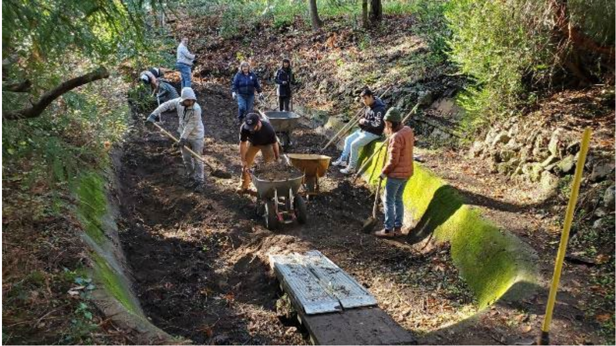
Figure 150. Excavating the lily ponds that were built by the Duvenecks near their house.
